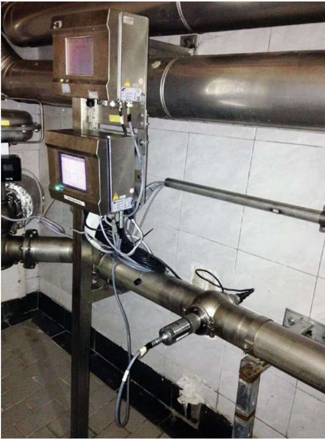
Figure 2: Hach 410 Controllers – typical installation
