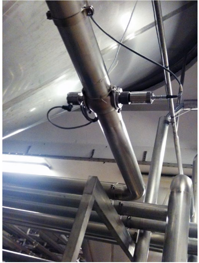
Figure 3: Hach M1100-H LDO Sensor – typical installation
